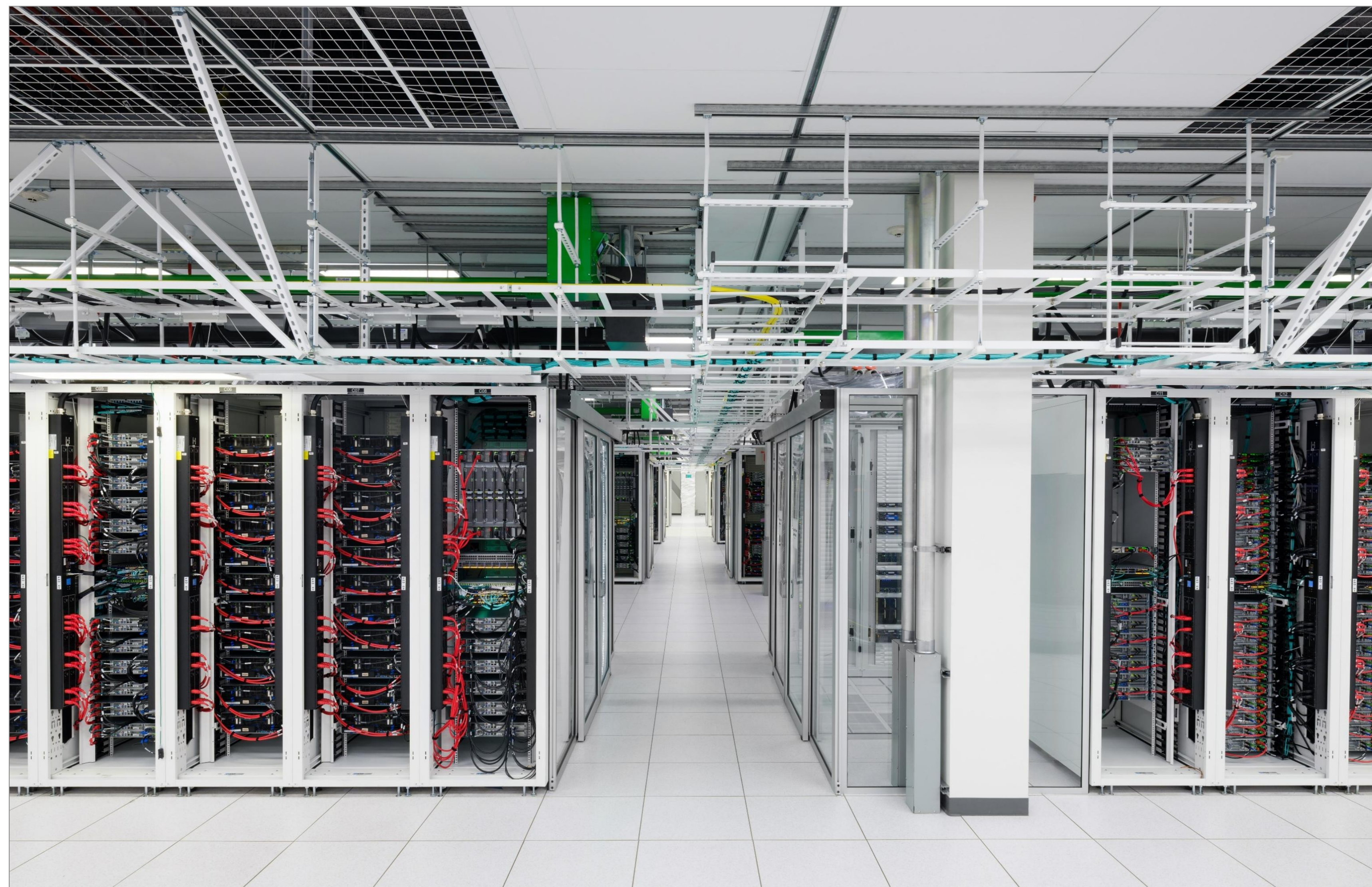
Traditional Cloud Data Center
